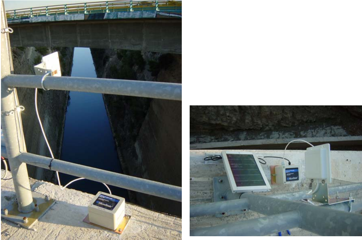
Figure 4-5. Solar powered wireless G-Link® seismic sensors on Corinth Bridge, Greece
