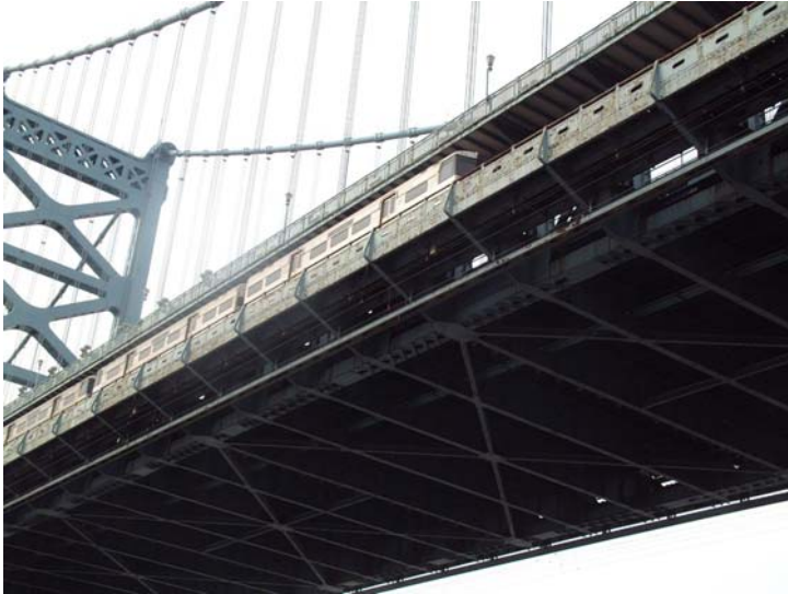
Figure 2. Passenger trains crossing the Ben Franklin bridge. Four wireless nodes were placed strategically at each end of the span. Each node autonomously collected data from three distinct strain gauges per node (for 12 total strain measurements). Temperatures were also monitored at each node location.
